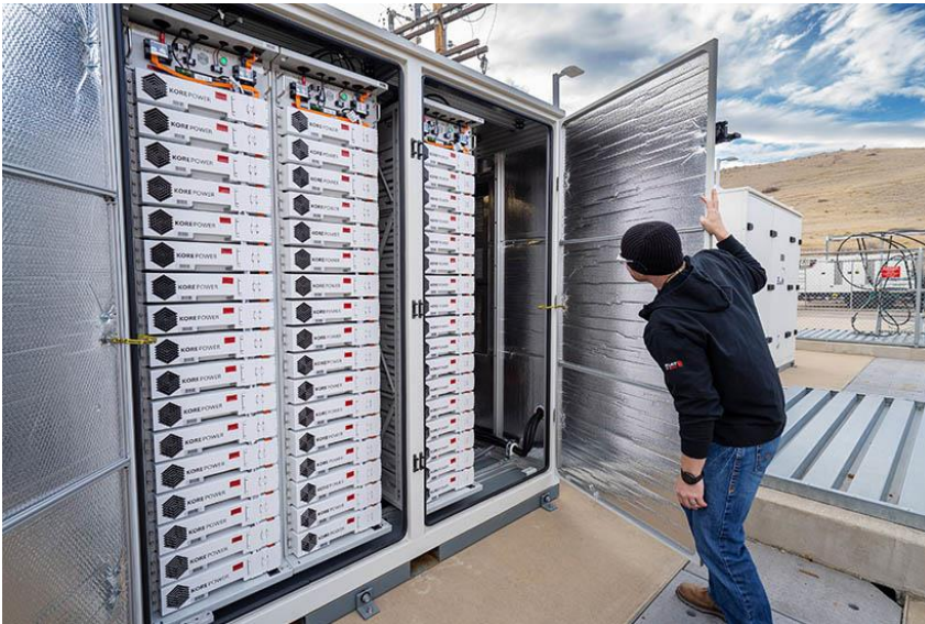
Figure 5 BESS access from the outside (Source: NREL)
